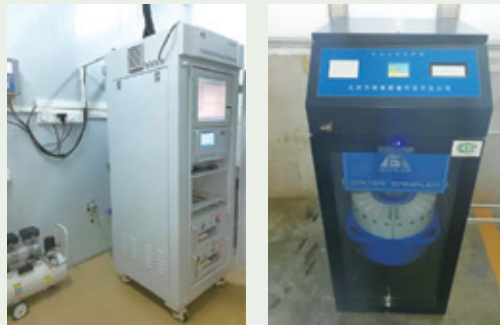
Automatic sampling and monitoring system for wastewater and exhaust gas
